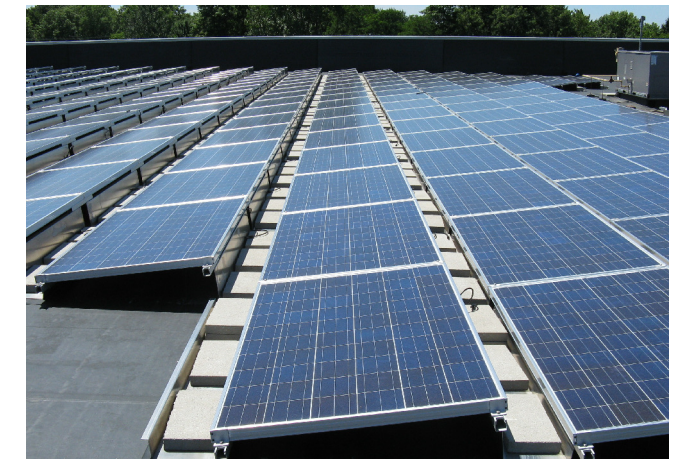
PHOTO SOURCE - © 2010 BIRDSALL SERVICES GROUP NOTE: ROOFS OF THIS BUILDING ARE COAL TAR
