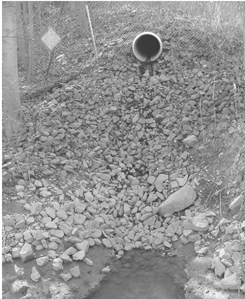
A scour hole is caused by excessive velocity of the discharge. Riprap may help dissipate the flow, reducing damage to the stream bank.
