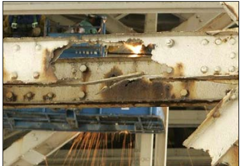
A rusted support beam of the 12th and 14th St. Viaduct in Jersey City, N.J. (October 2007)
